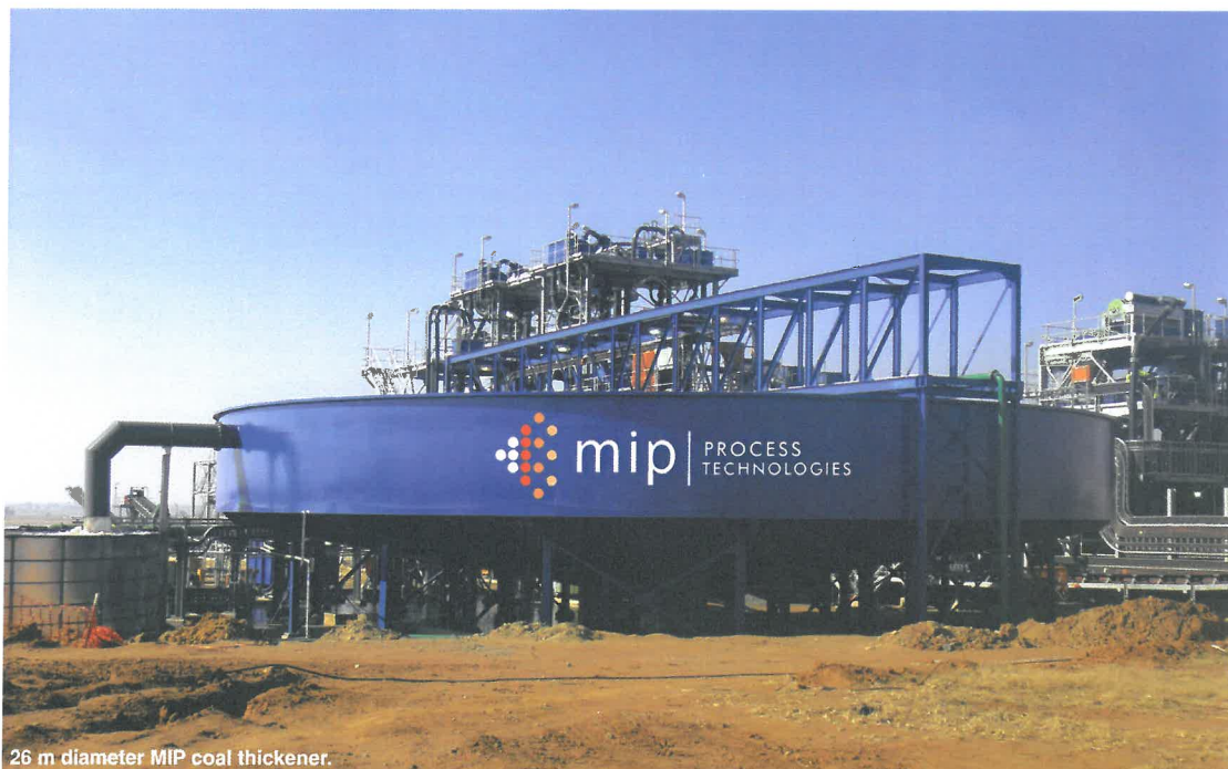
26 m diameter MIP coal thickener.
