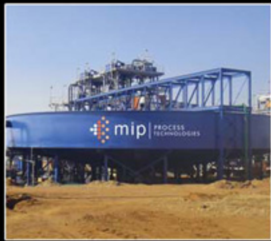
26m \phi Thickener in operation
